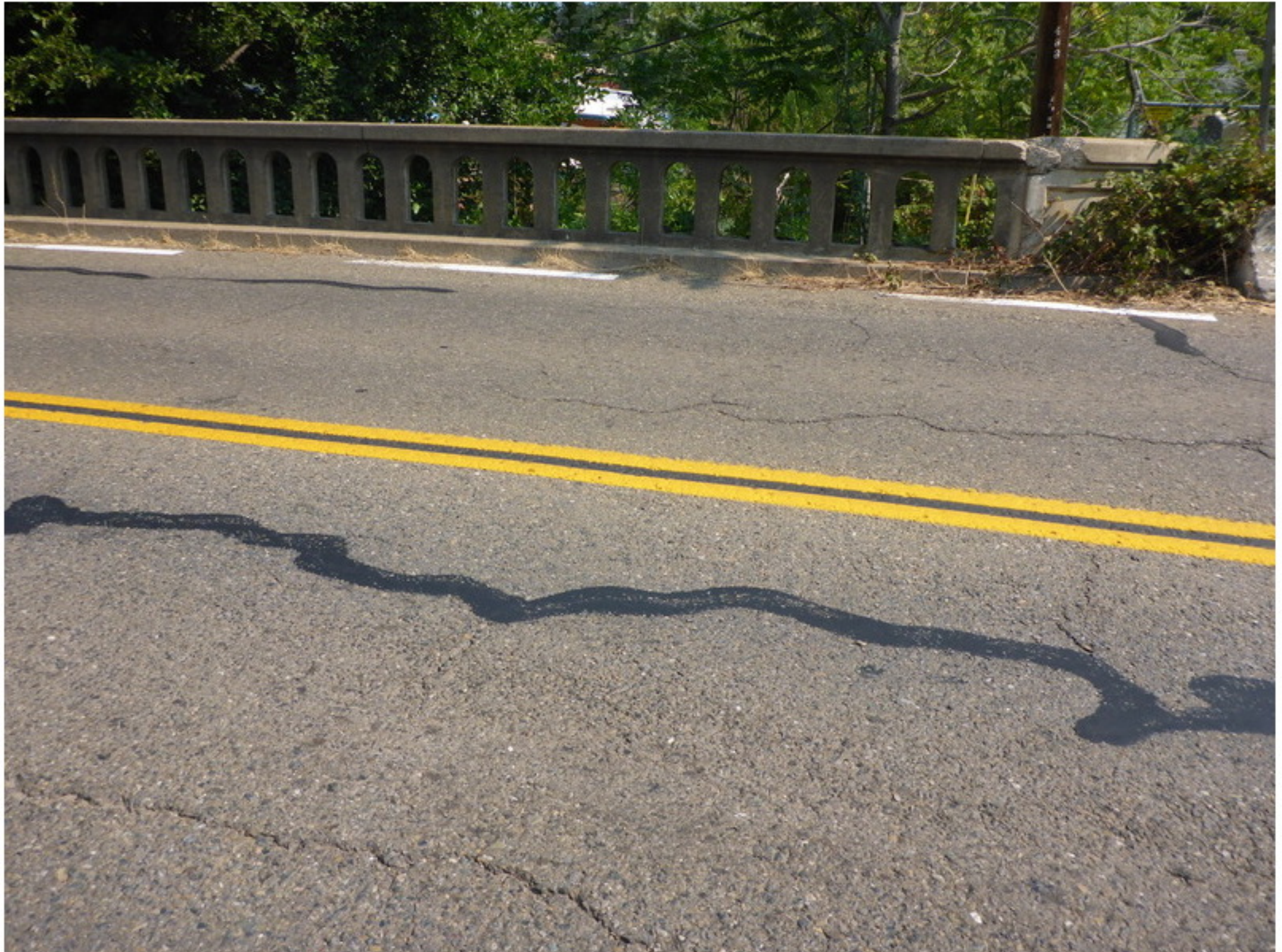
Photo No. 7 Longitudinal cracks in AC
