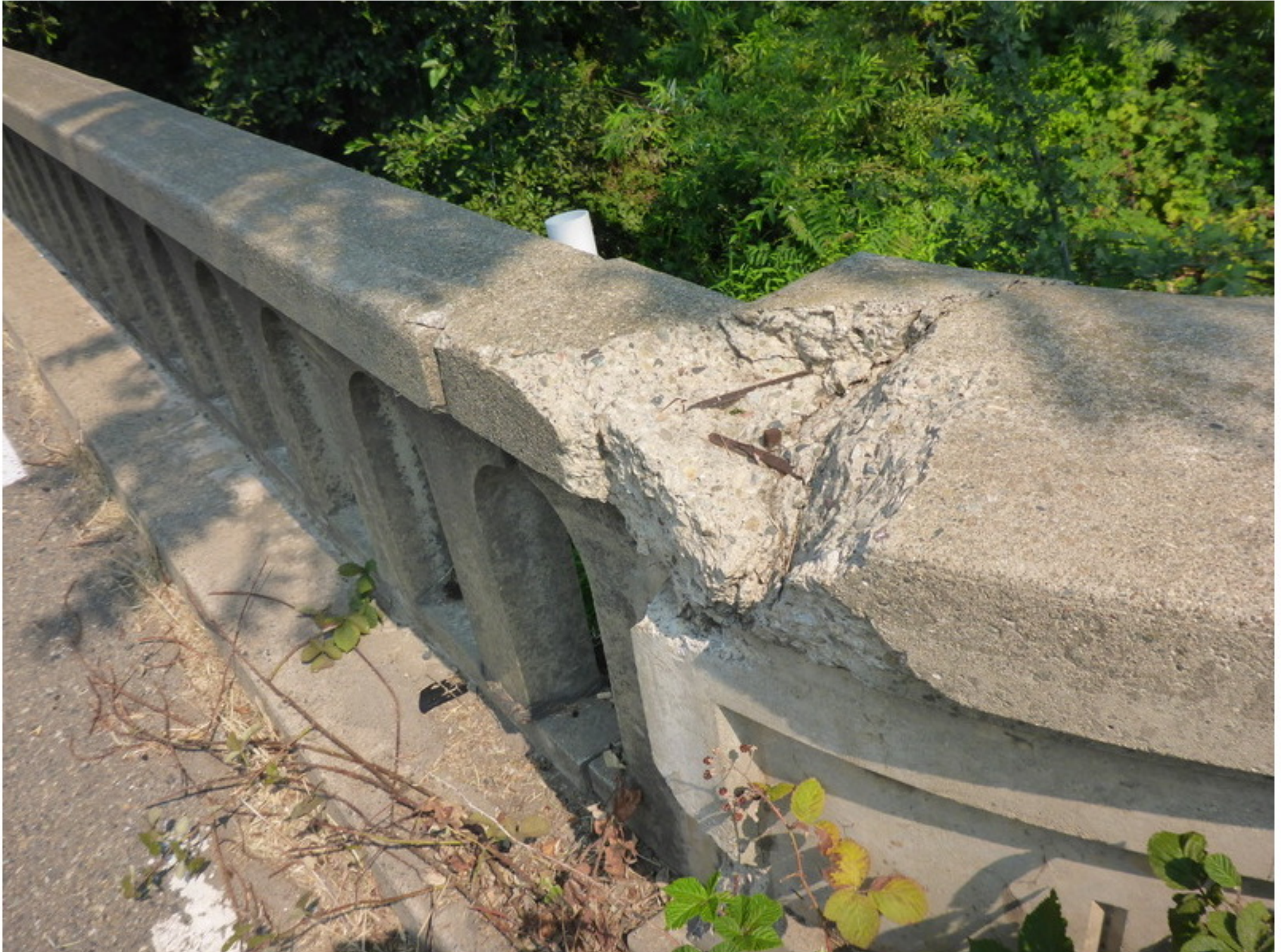
Photo No. 6 18 inch diameter rail spall at left side of Abutment 2
