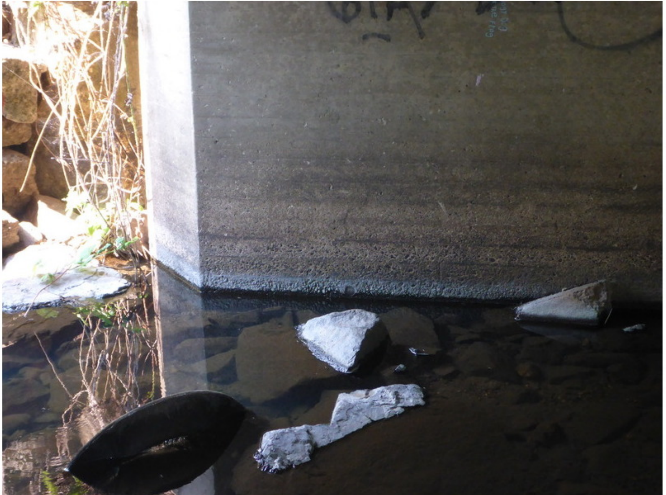
Photo No. 4 Abrasion on right half of Abutment 1
