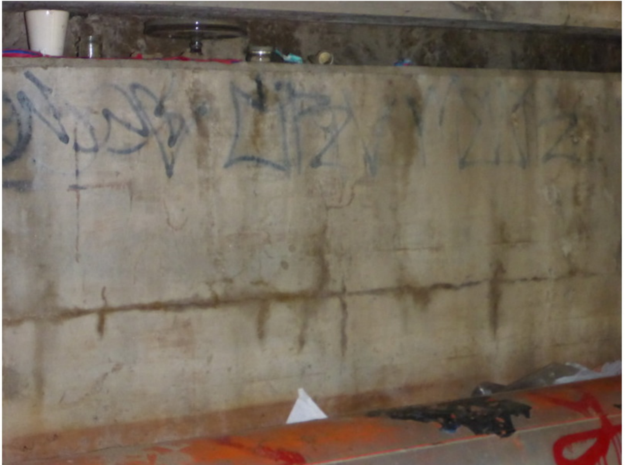
Photo No. 5 Horizontal crack along Abutment 2
